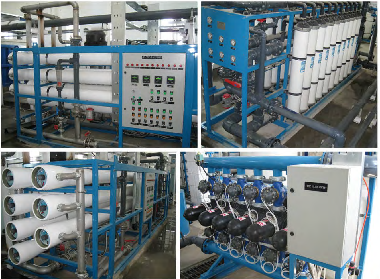
Complete Design and supply of one 1000 m 3 /day BW RO Unit – Ruhubelent, Turkmenistan
