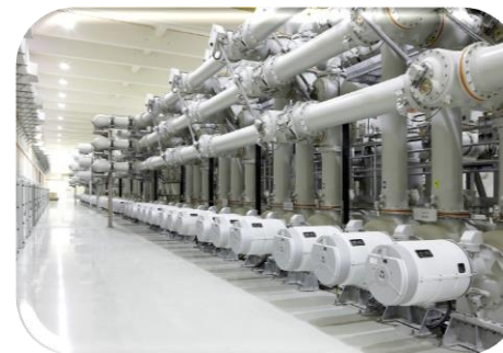
Gas Insulated Switchgears (GIS)
